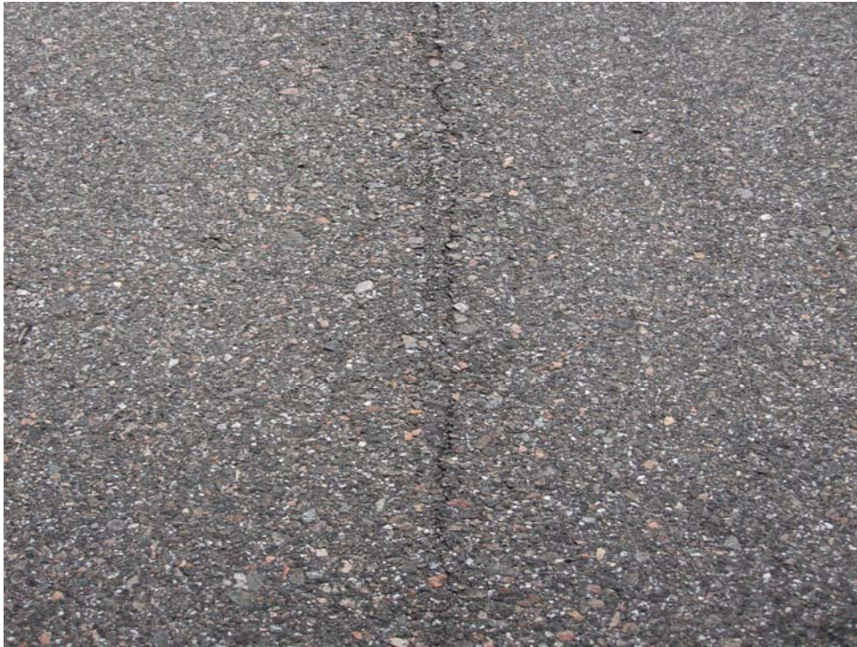
TCAGR-30. Longitudinal and Transverse Cracking (Sample Unit #26).
