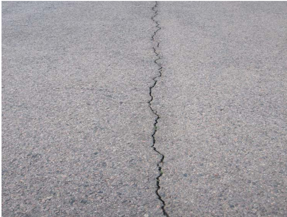
A01AGR-40. Longitudinal and Transverse Cracking (Sample Unit #15).
