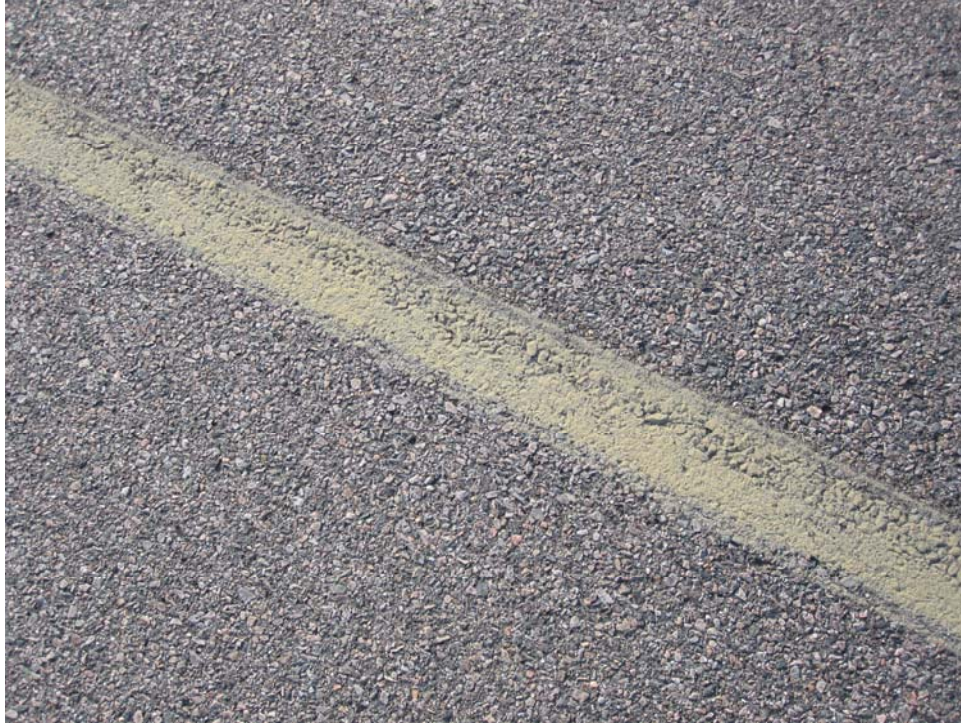
AGARRETAGR-20. Unsatisfactory Paint.
