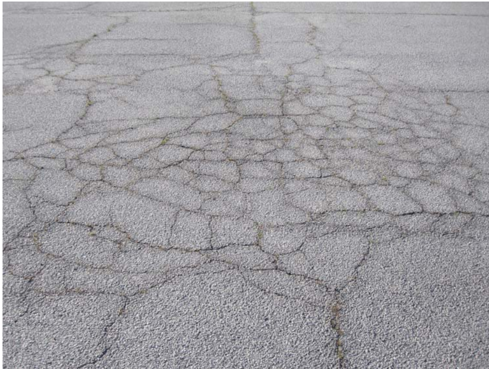
AGARRETAGR-40. Alligator Cracking (Sample Unit # 08).
