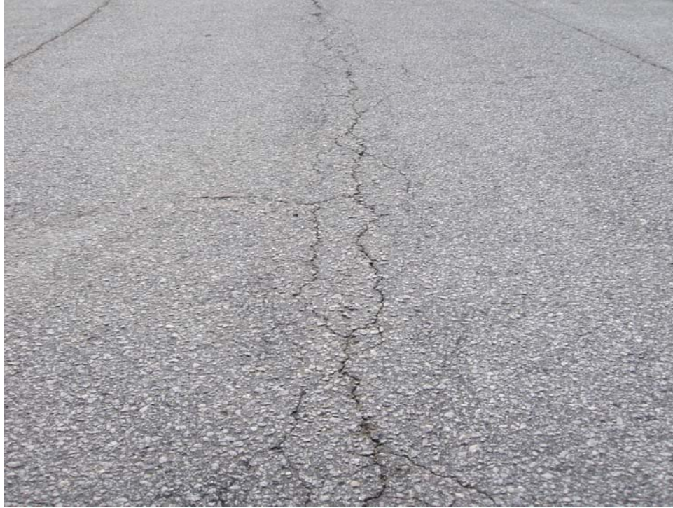
TAAGR-20. Alligator Cracking (Sample Unit #37).
