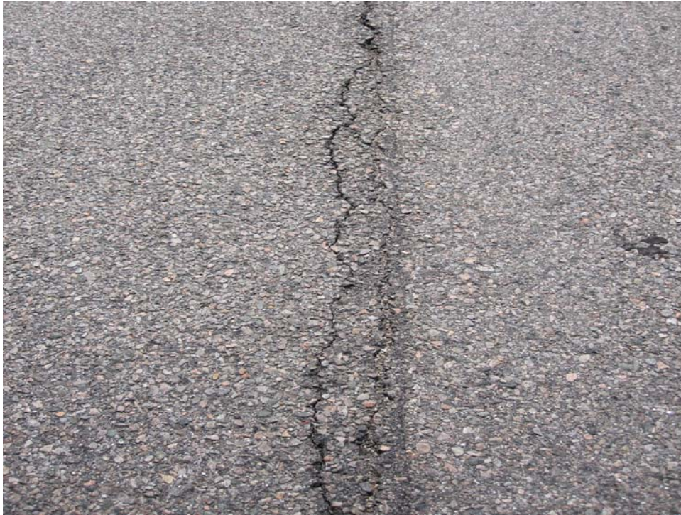
TCAGR-20. Longitudinal and Transverse Cracking (Sample Unit #25).
