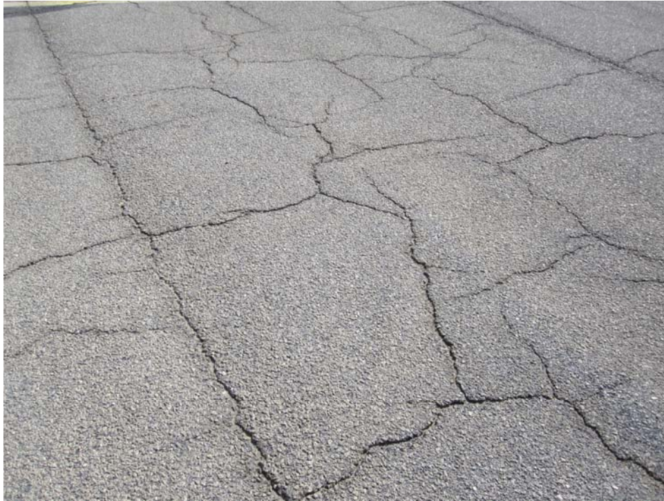
A01AGR-30. Block Cracking (Sample Unit #17).
