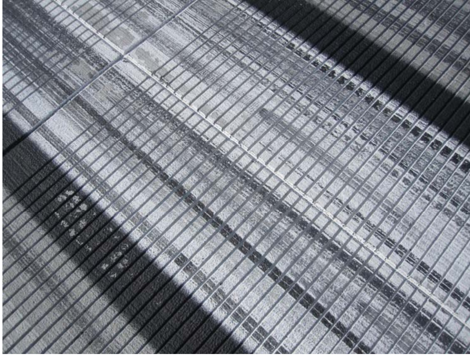
R1735AGR-20C. Satisfactory Paint.
