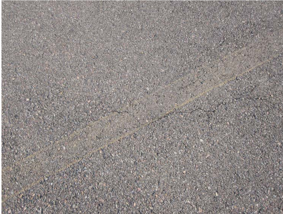
A01AGR-60. Unsatisfactory Paint.
