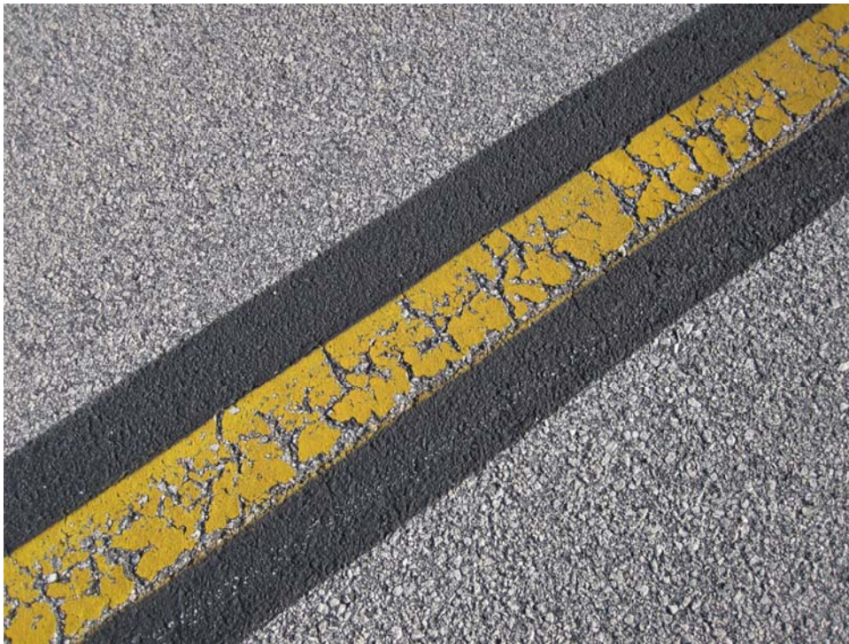
TEAGR-20. Unsatisfactory Paint.
