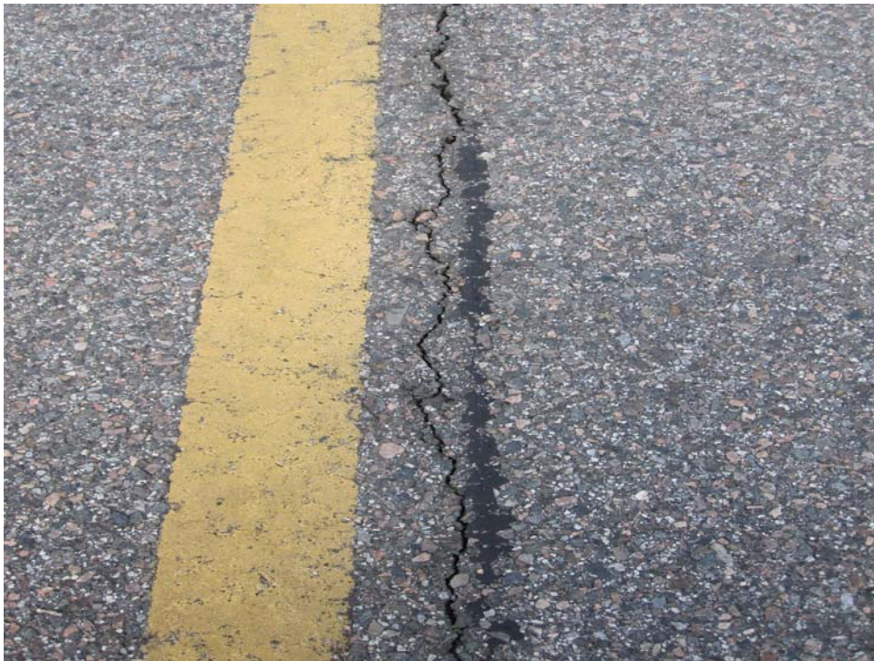
TCAGR-30. Bleeding (Sample Unit #22).
