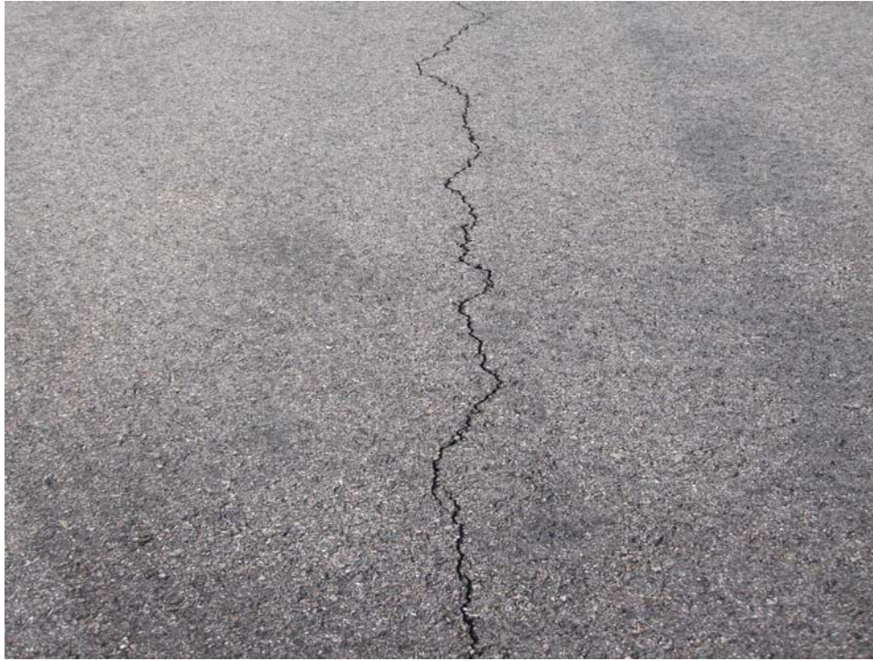
A01AGR-70. Longitudinal and Transverse Cracking (Sample Unit #03).
