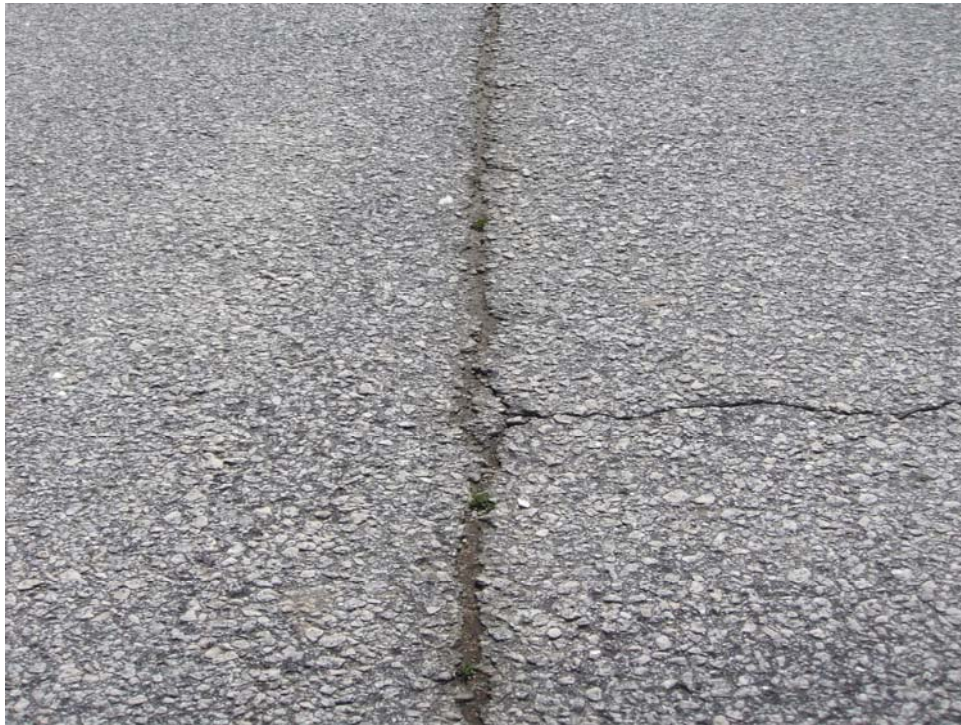
TAAGR-20. Longitudinal and Transverse Cracking (Sample Unit #32).
