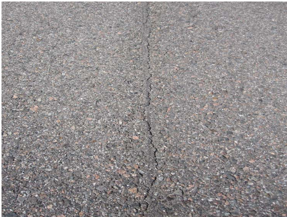
HELIAGR-10. Longitudinal and Transverse Cracking (Sample Unit #03).
