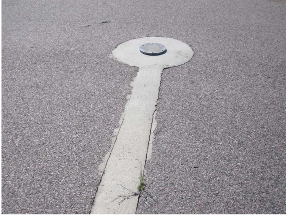
R0826AGR-10. Patching (Sample Unit #02).
