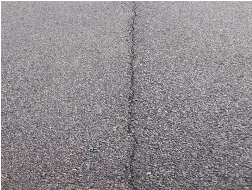
AGARRETAGR-20. Longitudinal and Transverse Cracking (Sample Unit #02).
