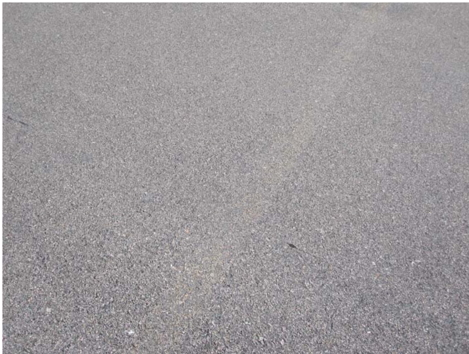
A01AGR-70. Unsatisfactory Paint.
