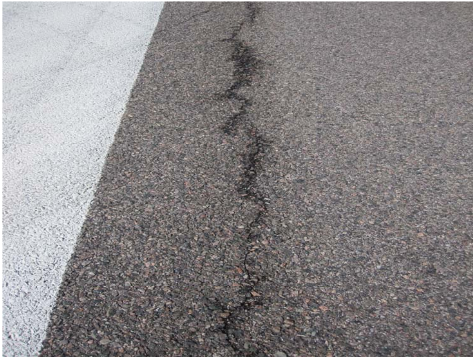
R0826AGR-10. Longitudinal and Transverse Cracking (Sample Unit #02).
