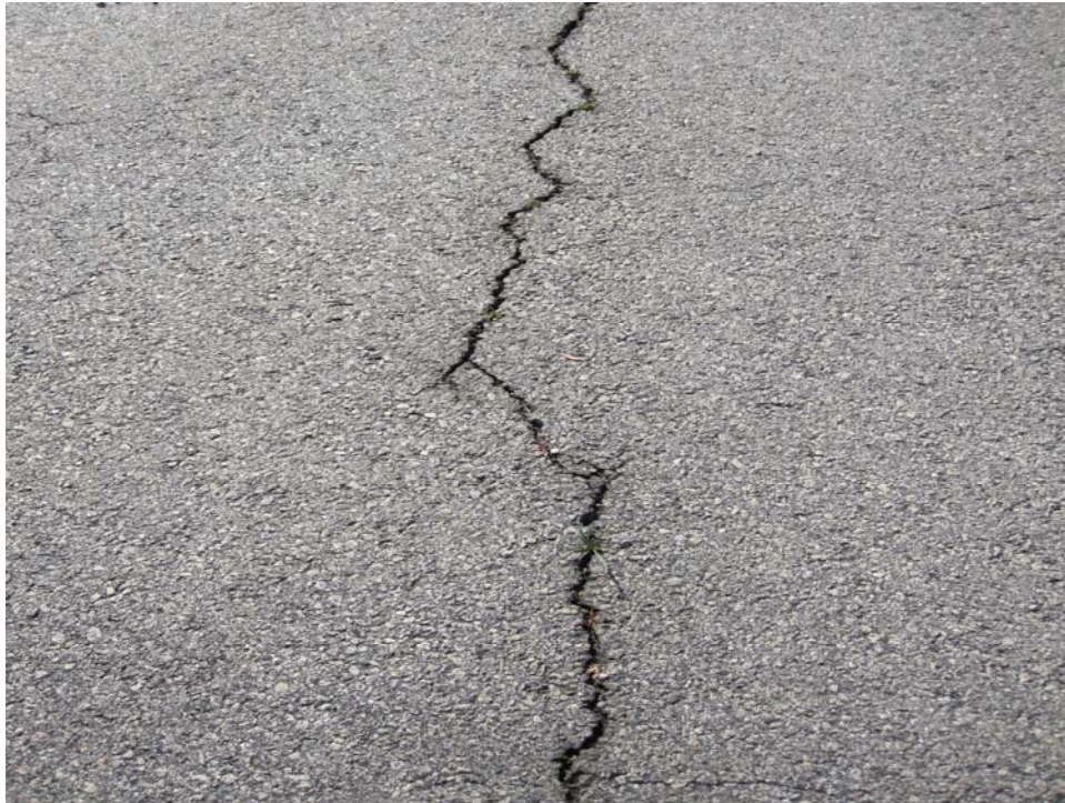
A01AGR-10. Longitudinal and Transverse Cracking (Sample Unit #05).
