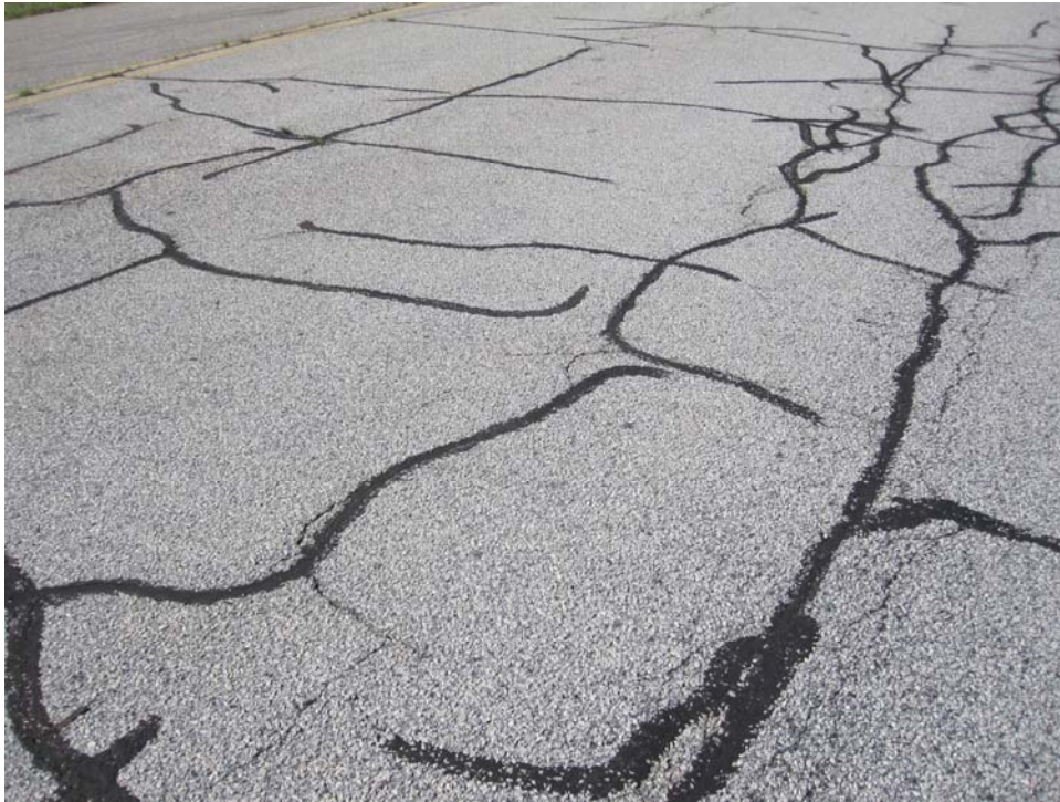
TEAGR-10. Block Cracking (Sample Unit #03).
