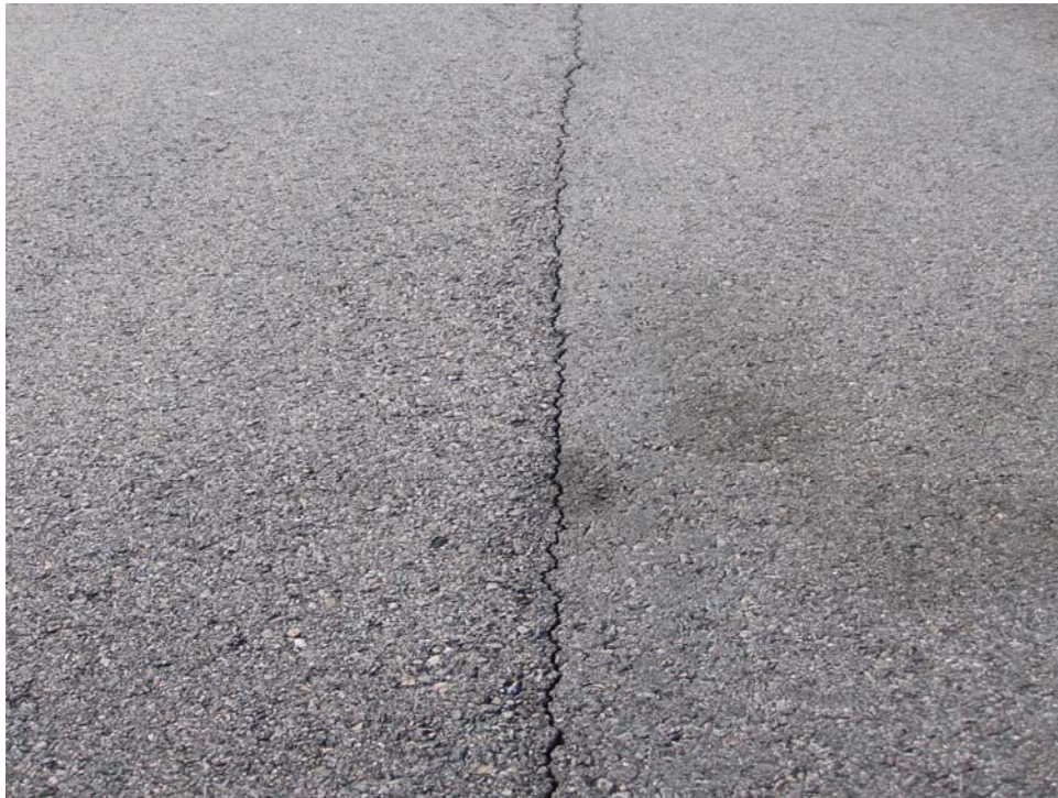
A01AGR-50. Longitudinal and Transverse Cracking (Sample Unit #08).
