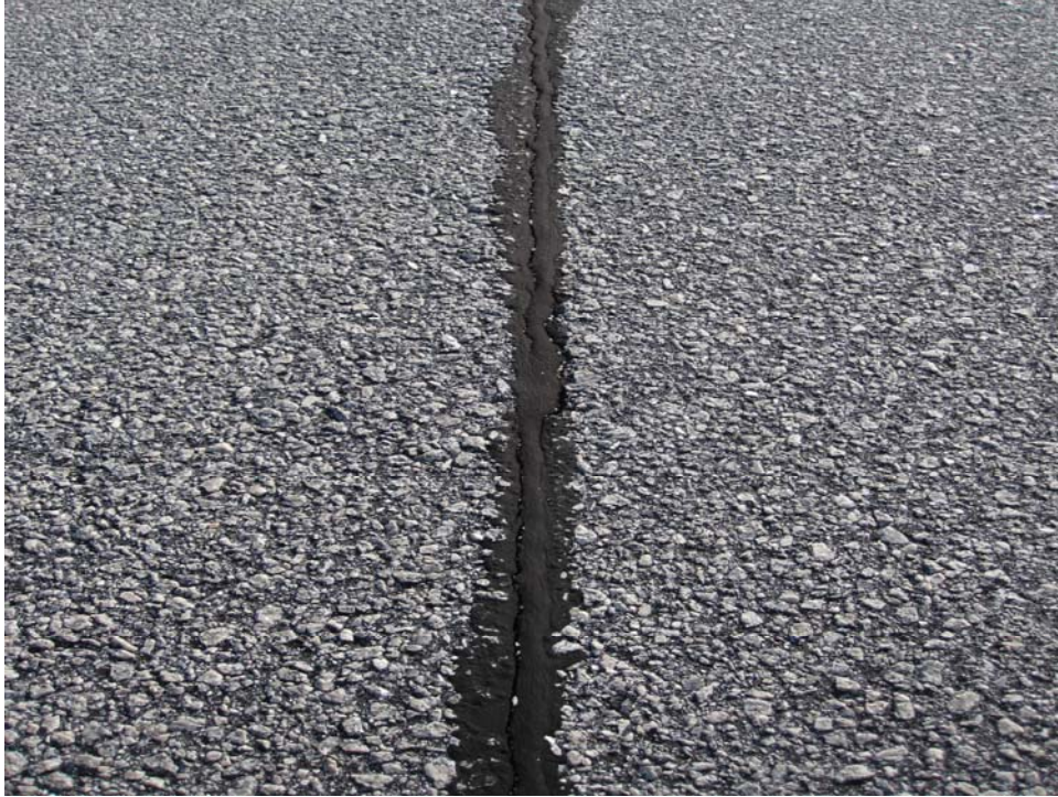
TEAGR-20. Longitudinal and Transverse Cracking (Sample Unit #44).
