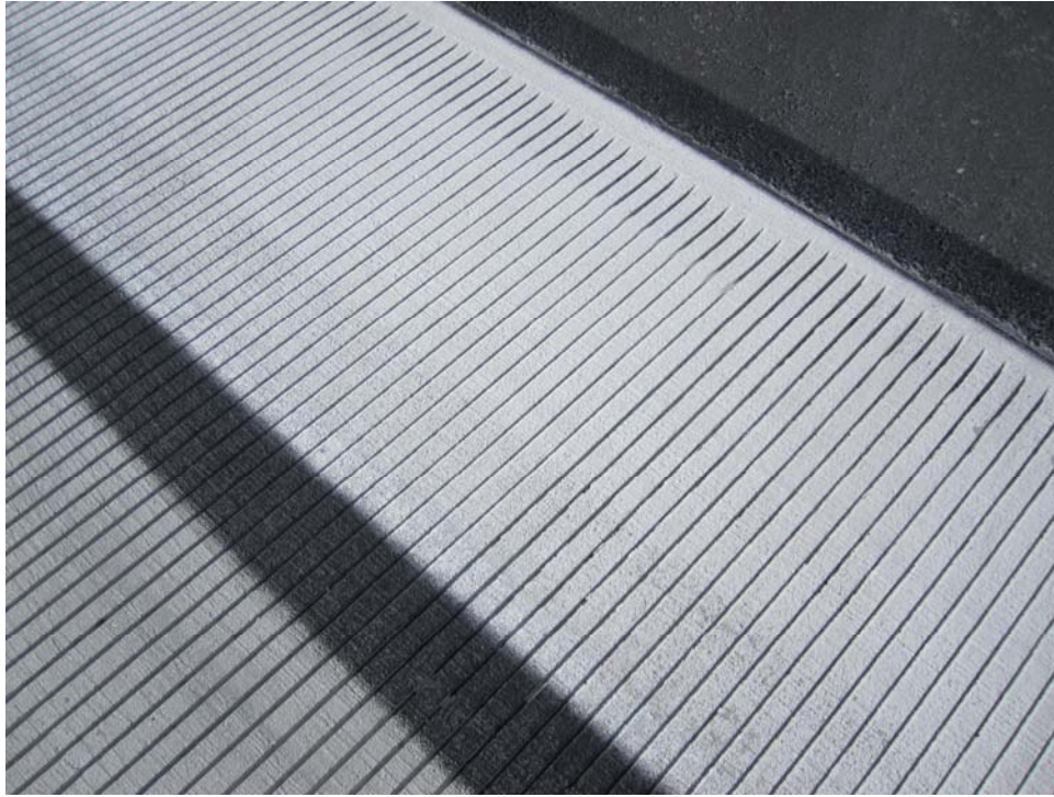
R1735AGR-20W. Satisfactory Paint.
