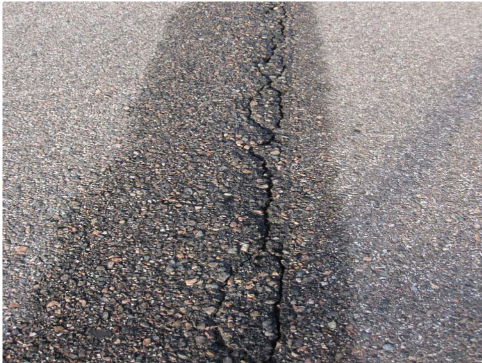
R0826AGR-30. Longitudinal and Transverse Cracking (Sample Unit #66).
