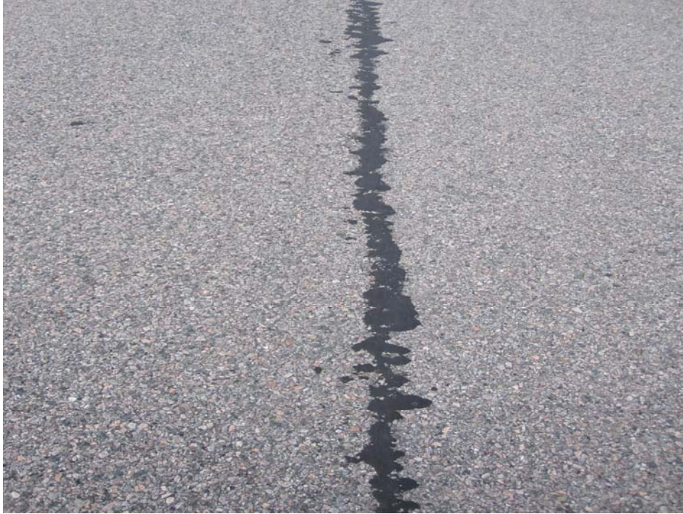
TCAGR-20. Bleeding (Sample Unit #40).
