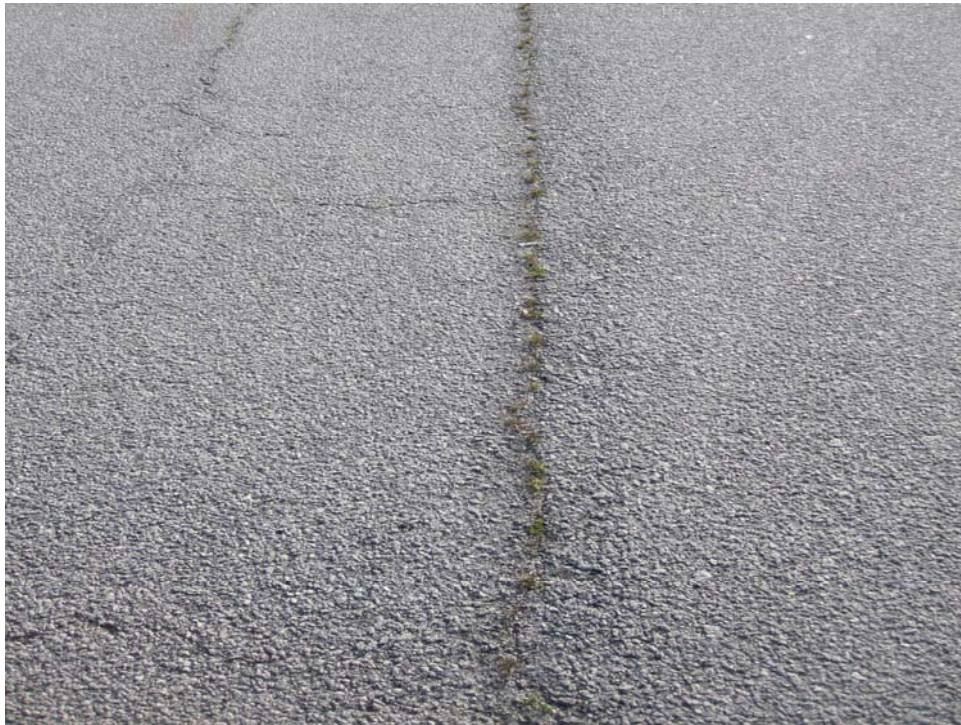
AGARRETAGR-40. Longitudinal and Transverse Cracking (Sample Unit #11).
