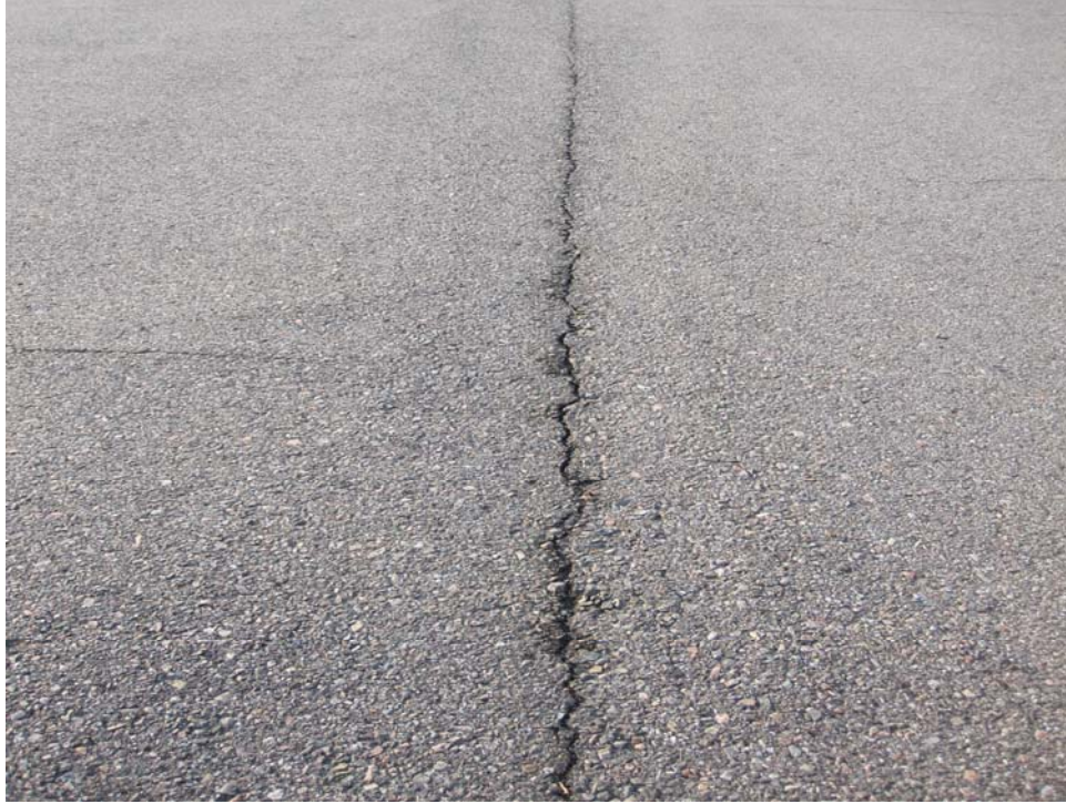
A01AGR-60. Longitudinal and Transverse Cracking (Sample Unit #13).
