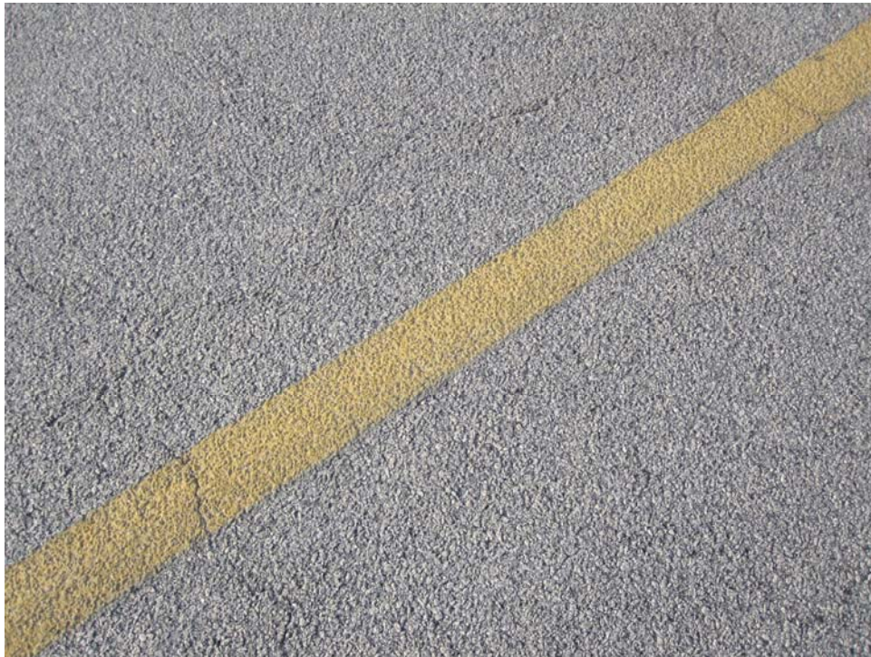
AGARRETAGR-30. Satisfactory Paint.
