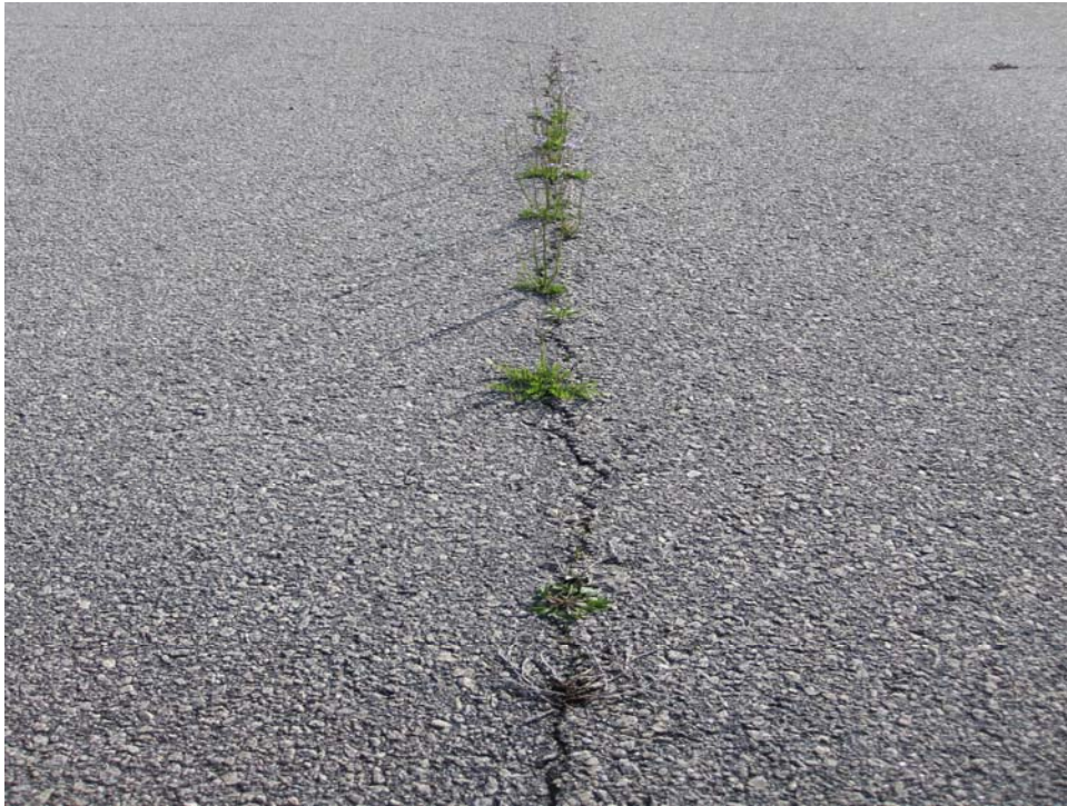
TEAGR-20. Longitudinal and Transverse Cracking (Sample Unit #36).
