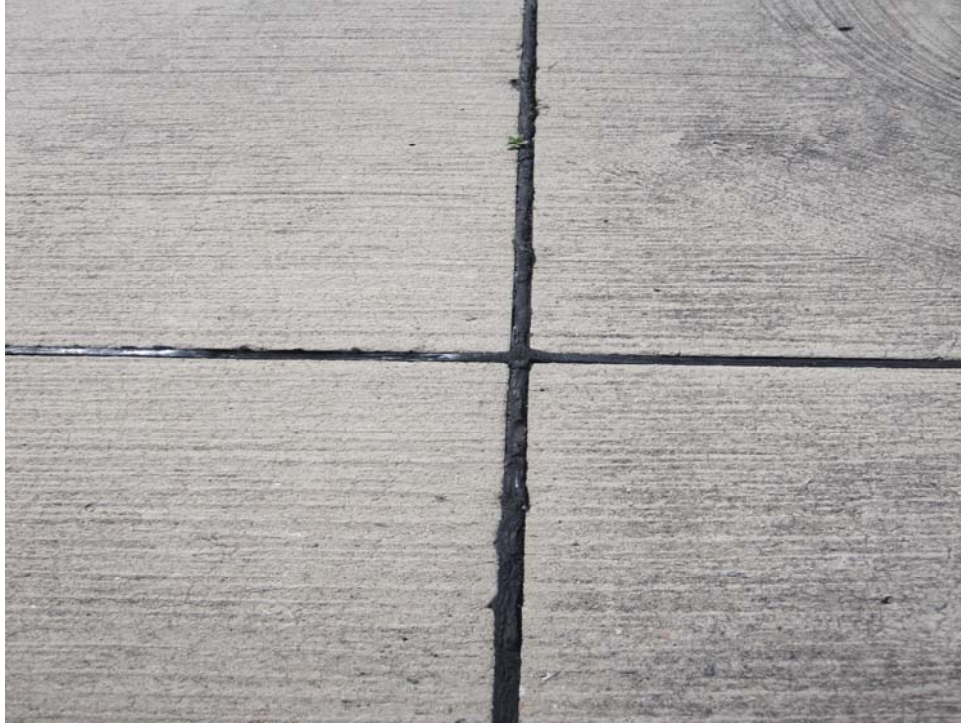
HELIAGR-20. Joint Seal Damage (Sample Unit #01).
