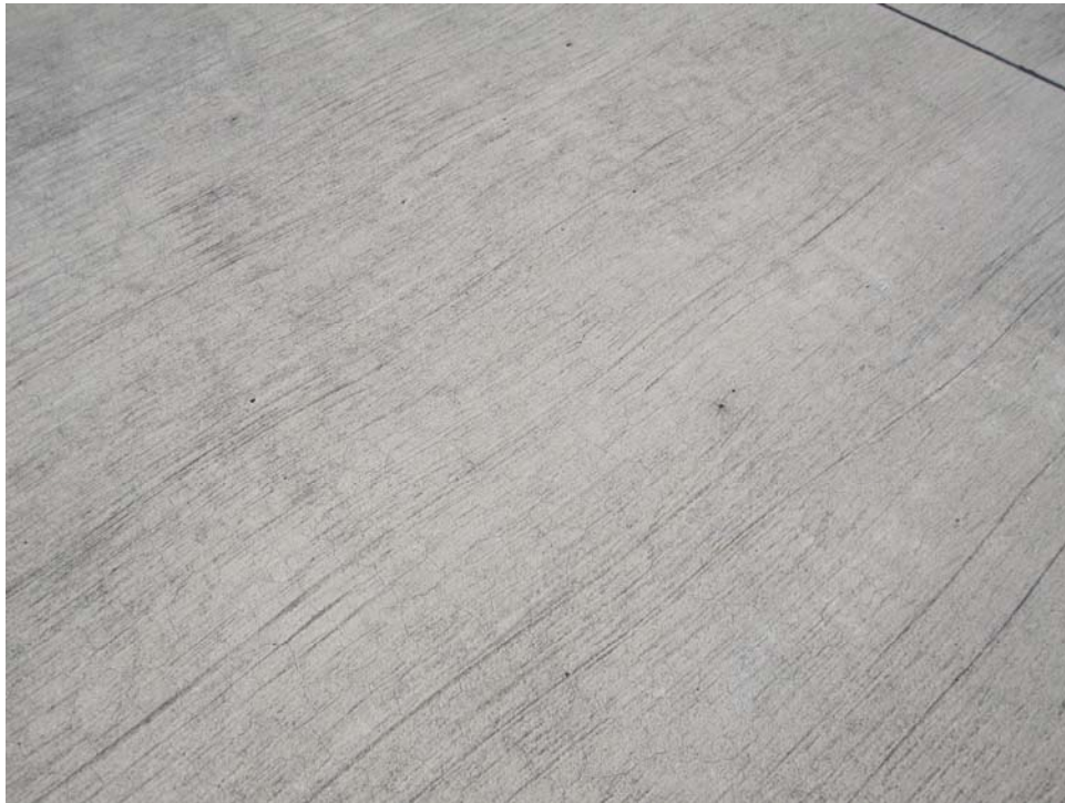
HELIAGR-20. Shrinkage Cracking (Sample Unit #02).
