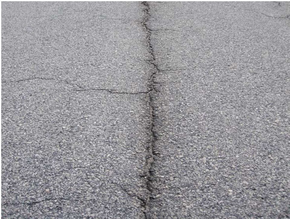
TCAGR-10. Longitudinal and Transverse Cracking (Sample Unit #01).
