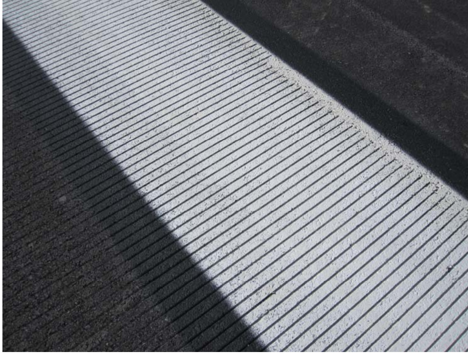
R1735AGR-10W. Satisfactory Paint.
