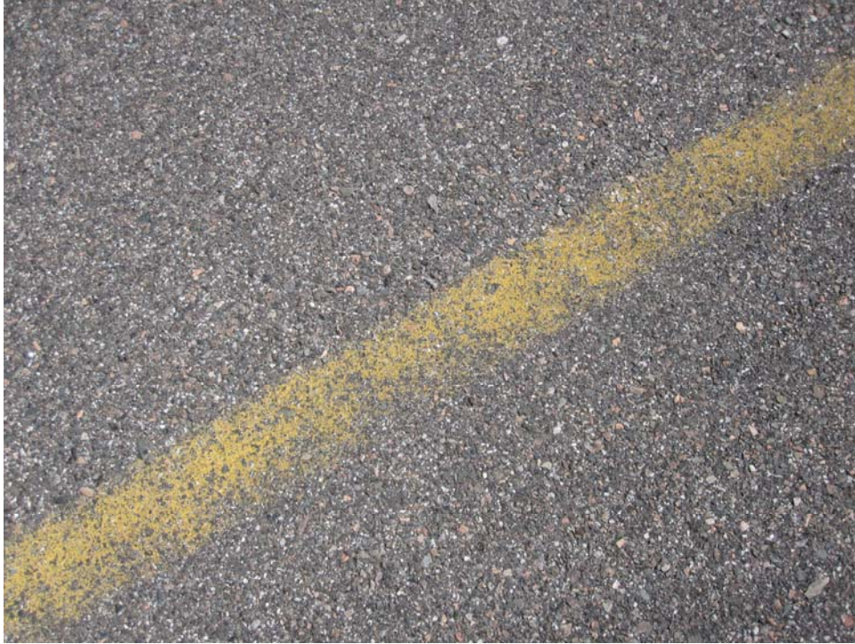
TCAGR-30. .Unsatisfactory Paint.
