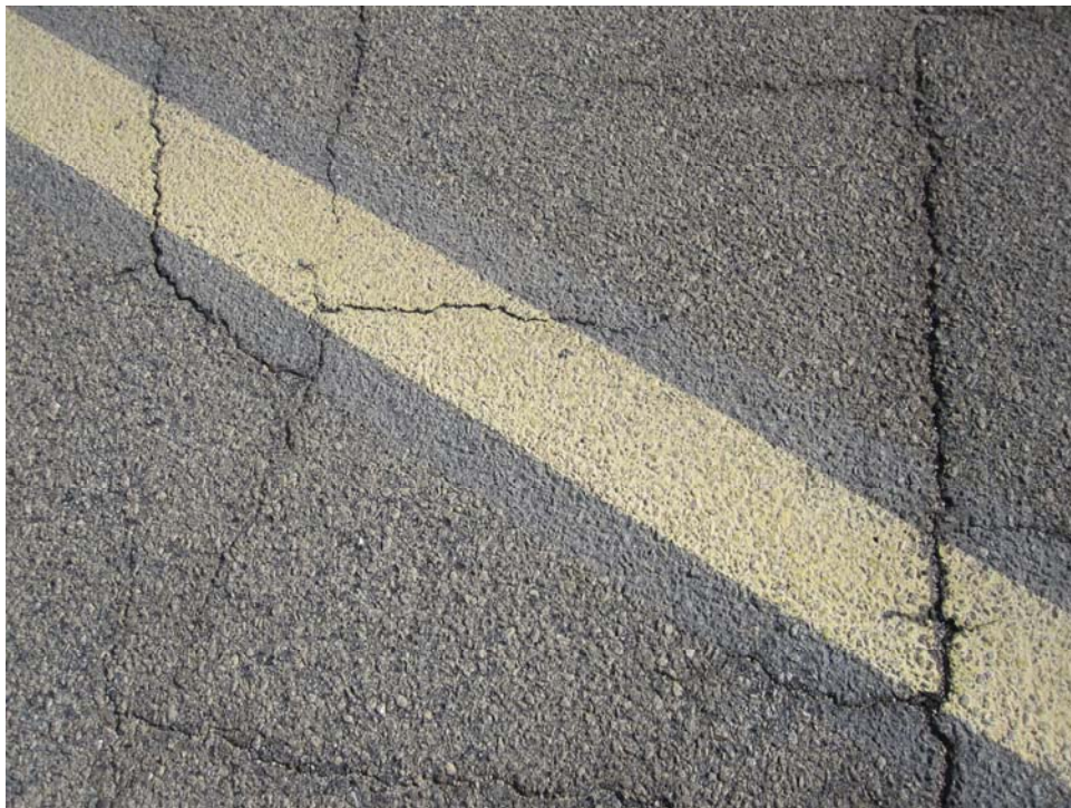
A01AGR-30. Unsatisfactory Paint.
