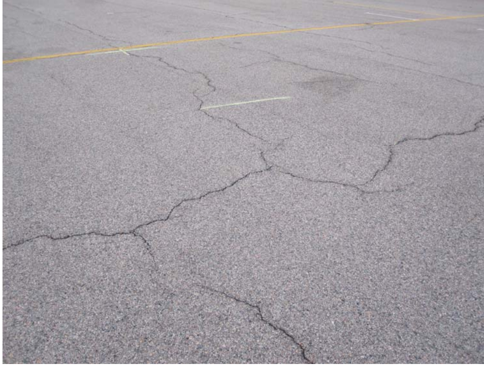
A01AGR-40. Longitudinal and Transverse Cracking (Sample Unit #41).
