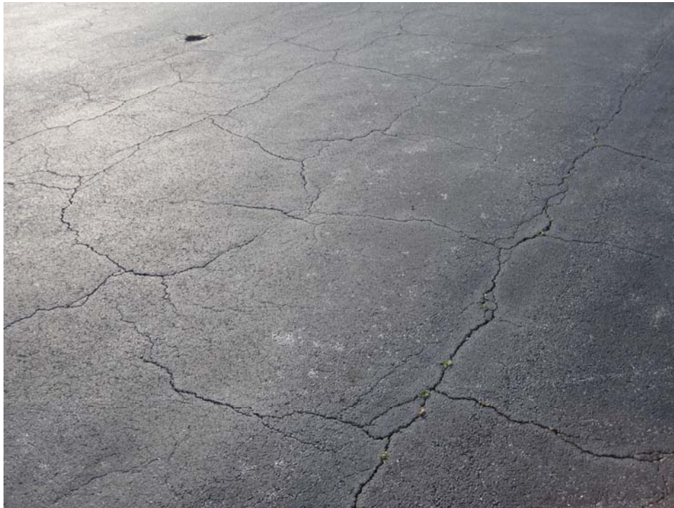
AGARRETAGR-10. Block Cracking (Sample Unit #06).
