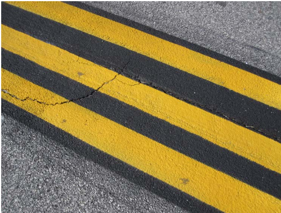
TBAGR-10. Satisfactory Paint.
