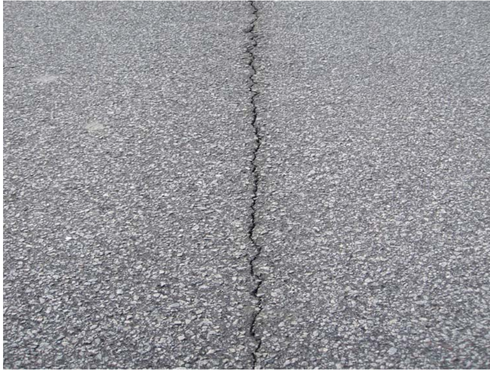
TDAGR-10. Longitudinal and Transverse Cracking (Sample Unit #07).
