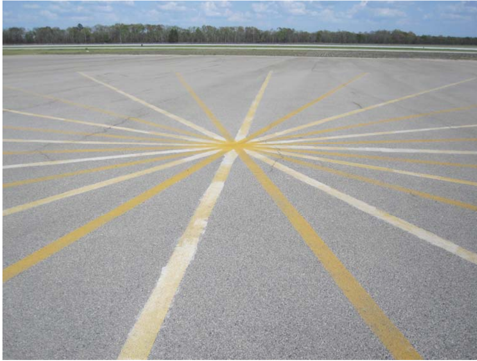
A01AGR-20. Unsatisfactory Paint.
