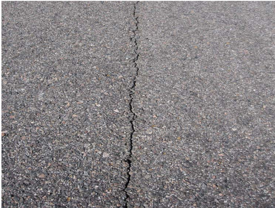
R0826AGR-20. Longitudinal and Transverse Cracking (Sample Unit #02).
