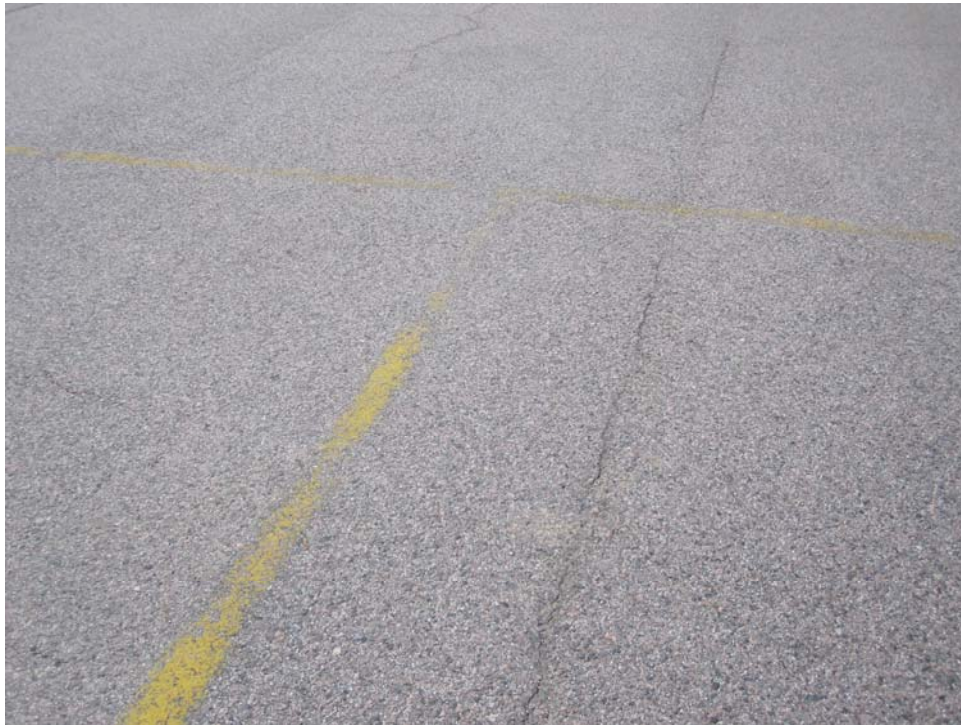
A01AGR-40. Unsatisfactory Paint.
