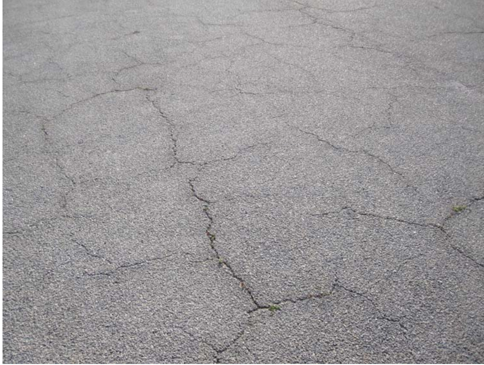
AGARRETAGR-30. Block Cracking (Sample Unit #05).
