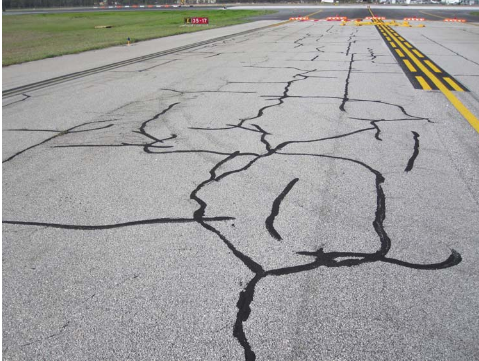
TEAGR-20. Longitudinal and Transverse Cracking (Sample Unit # 02).
