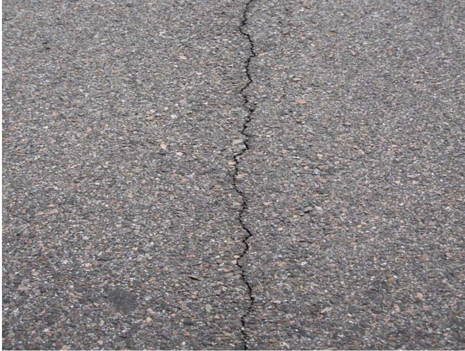
TCAGR-30. Longitudinal and Transverse Cracking (Sample Unit #22).
