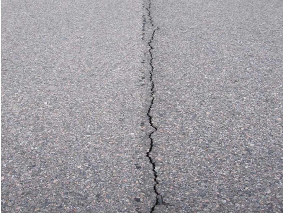
TCAGR-20. Longitudinal and Transverse Cracking (Sample Unit #35).
