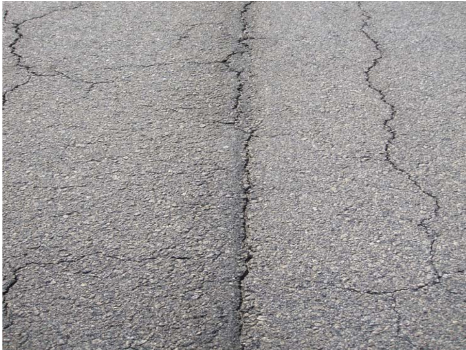
A01AGR-20. Longitudinal and Transverse Cracking (Sample Unit #12).
