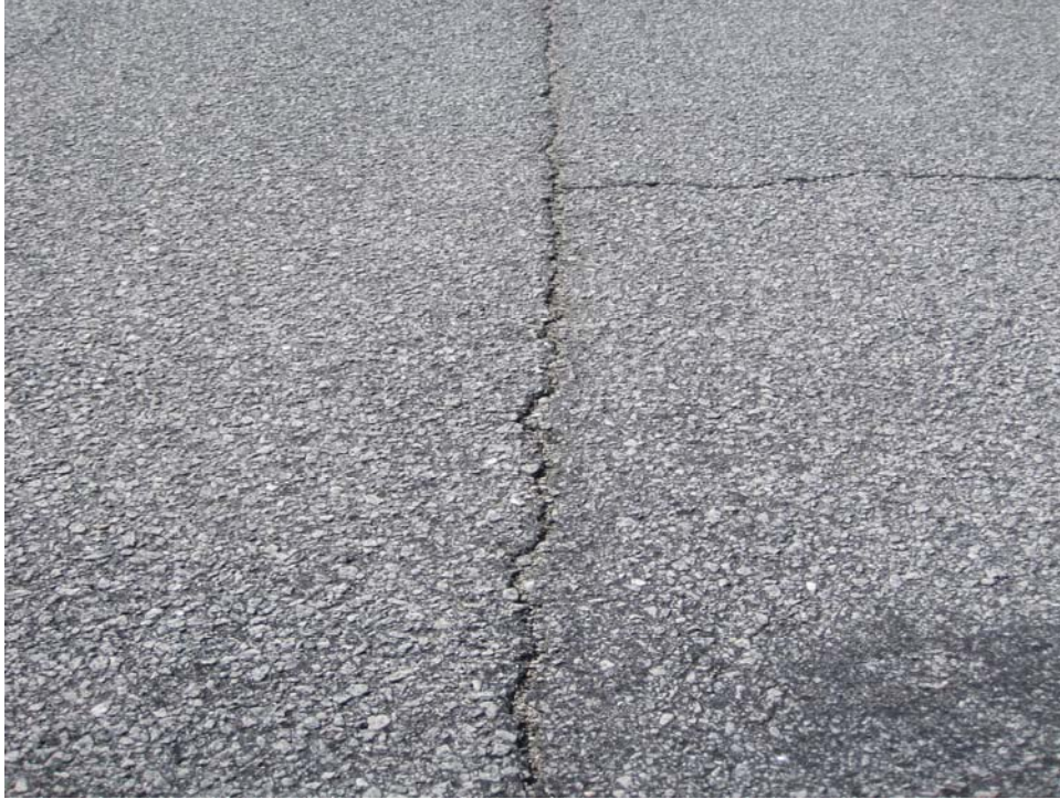
TBAGR-10. Longitudinal and Transverse Cracking (Sample Unit #06).
