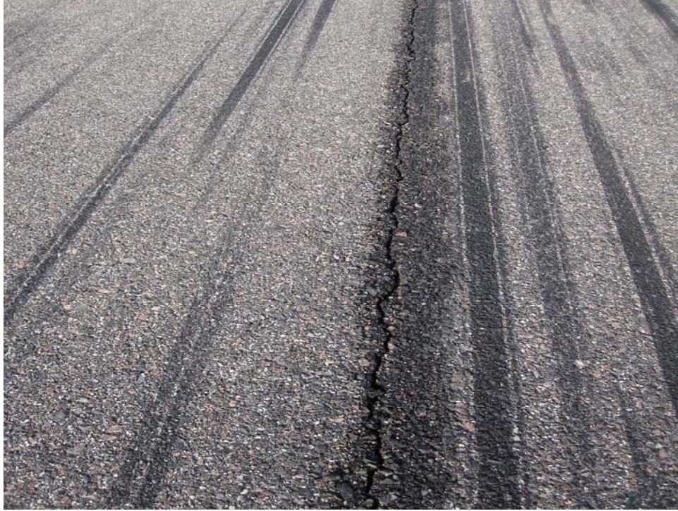
R0826AGR-30. Longitudinal and Transverse Cracking (Sample Unit #44).
