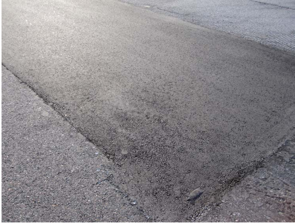
R0826AGR-30. Patching (Sample Unit #68).
