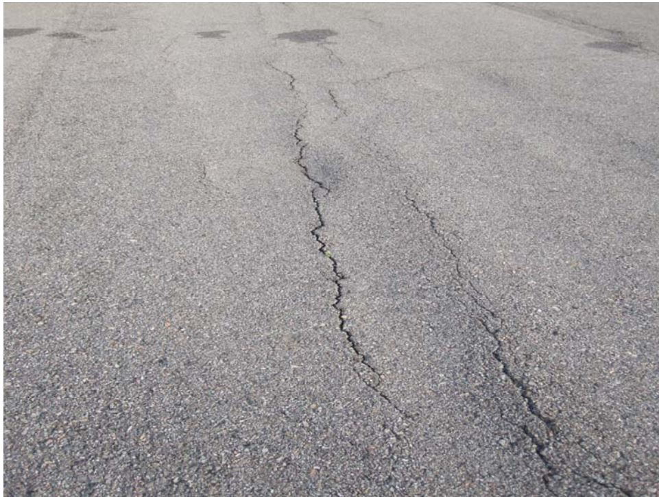
A01AGR-60. Rutting (Sample Unit #09).
